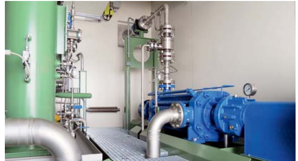
High-pressure injection skid with horizontal multistage pump
