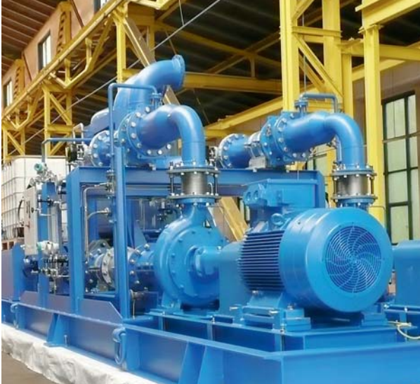
Transfer pump skid
